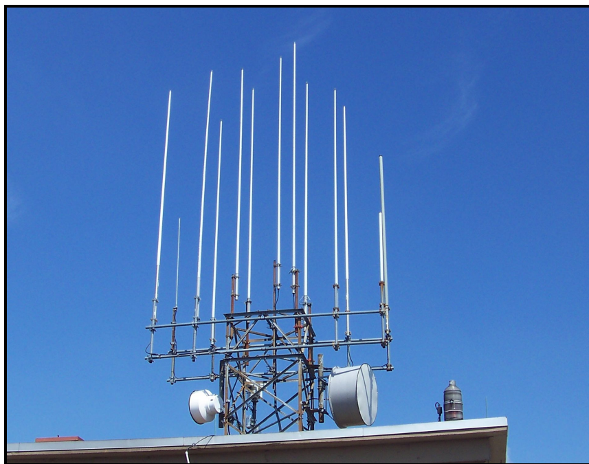
Antennas closely clustered on top of elevator penthouse
