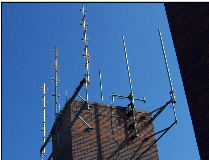
470 MHz and 800 MHz antennas in close proximity
